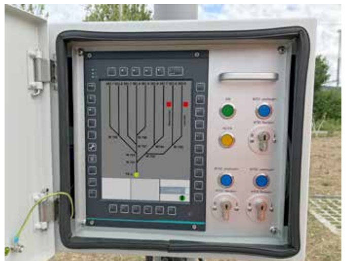
HPS Panel Station
