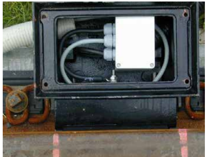
Blocking circuit terminal box
