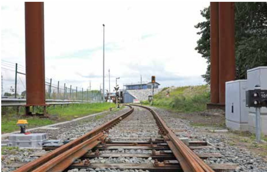
Electric locally-set point HN-EOW
