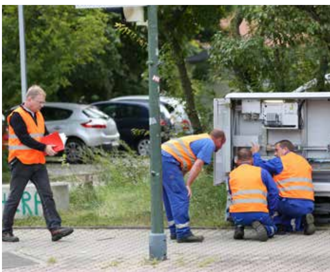
Regular preventative maintenance ensures trouble-free operations
