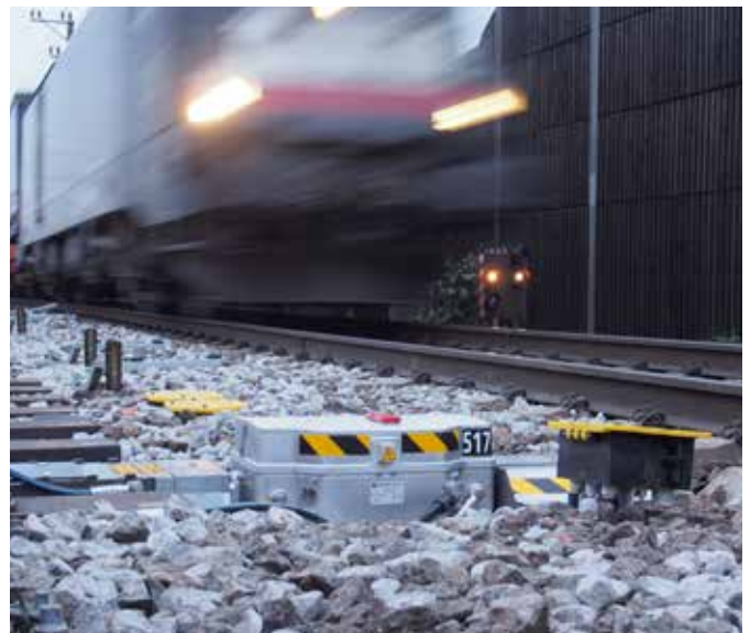
Point machine H715 installed in a main line
