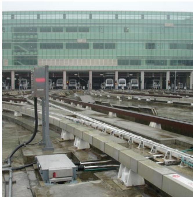
Point machine for the People Mover
